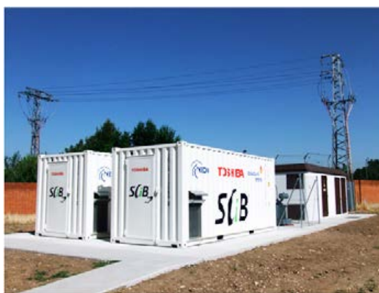
Figure 1-4 Energy storage system installed at a substation in Spain Source: http://www.nedo.go.jp/news/press/AA5_100459.html
