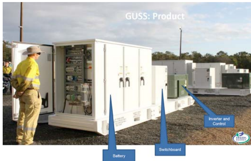
Figure 3-1 Grid Utility Storage System in Queensland, Australia Source: Ergon Energy
