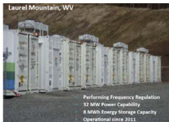
Figure 2-3 Batteries at Laurel Mountain installation Source: NEC Corporation
