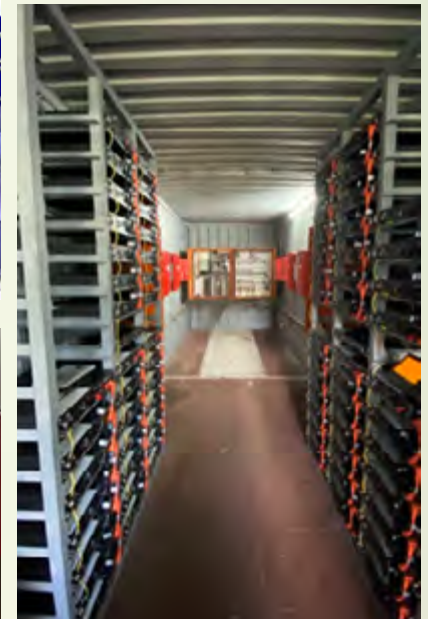
48 kWh Lithium ion battery and BMS
